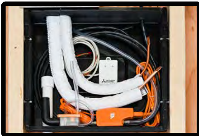
Piping connections and ancillary devices inside the box
